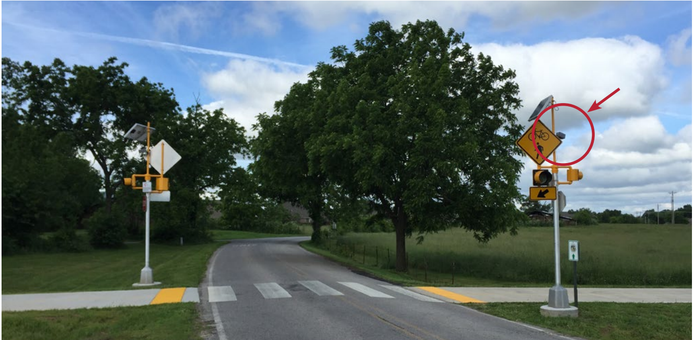
This microwave detector in along the Razorback Greenway in Northwest Arkansas activates a warning beacon when a trail user (pedestrian or bicyclist) is approaching the roadway crossing.
