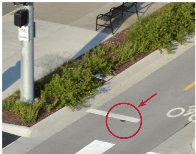
In-ground radar installation patch in Lincoln, NE. Ultimately, this system was deactivated and the signals reverted to fixed timing.
