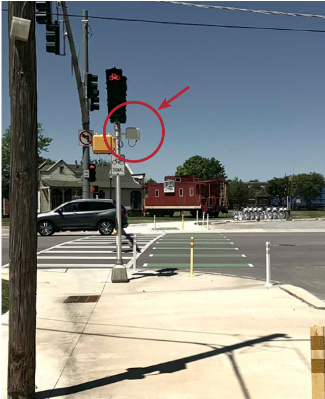
This microwave detector in Huntsville, AL, calls the bicycle signal only for approaching bicyclists who are within the separated bike lane. Microwave detectors can determine if the bicyclist is approaching or moving away from the intersection to avoid false calls.
