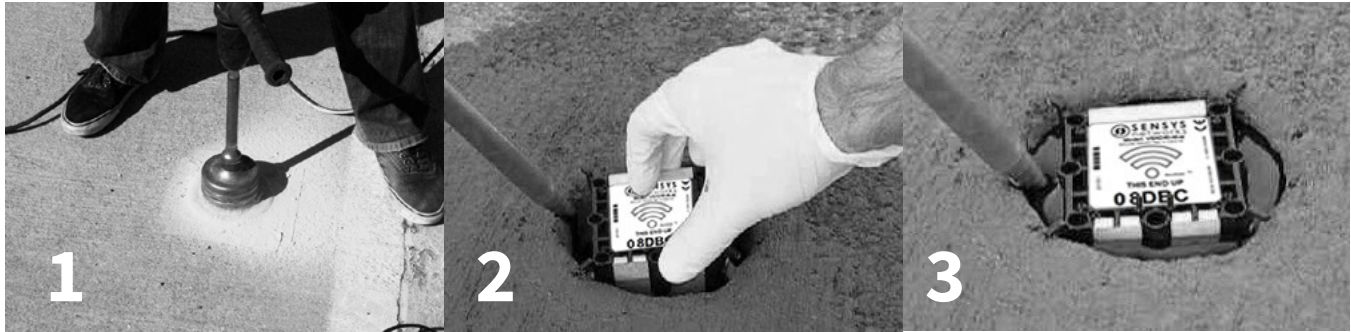
Installation includes (1) coring out a hole in the pavement, (2) placing the sensor, and (3) backfilling with epoxy
