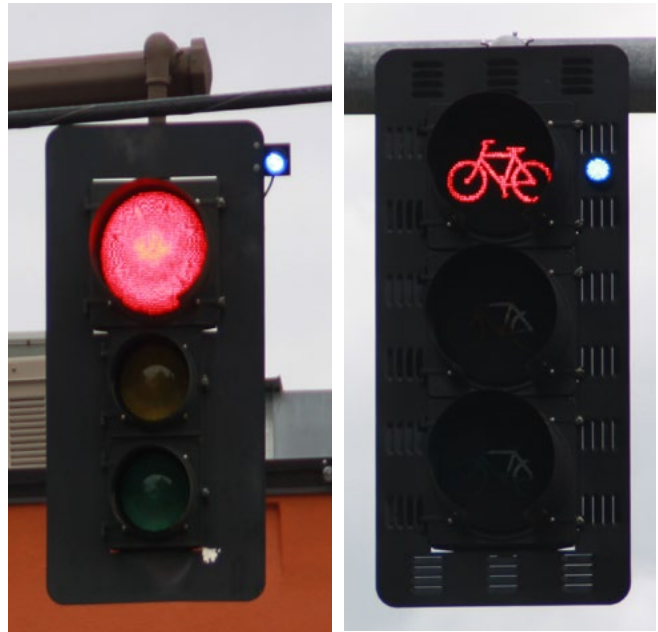
2012 and 2017 installations of blue lights integrated with signals
