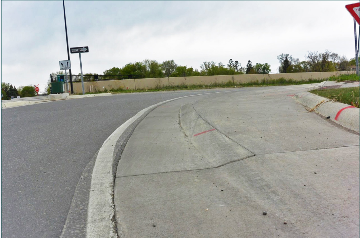
BELOW: A close-up view of the same channel showing the traversable curb profile.
