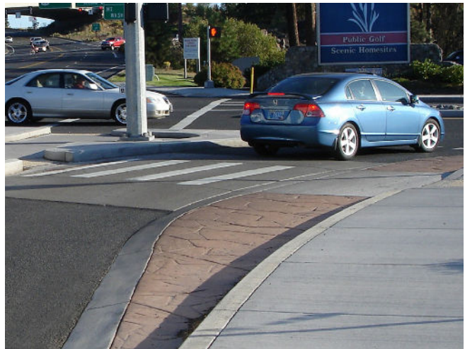
Crosswalk does not continue across mountable apron (Bend, OR)
