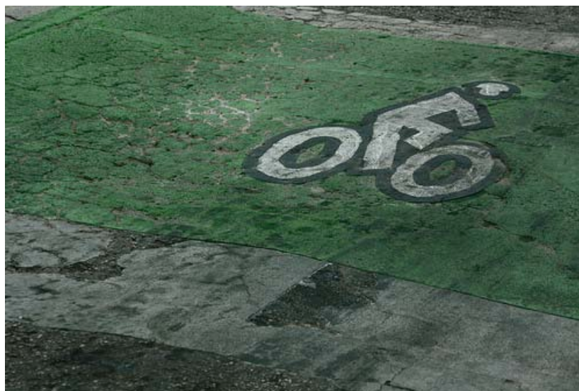
Figure B2. Poor quality of road lead to the deterioration of the thermoplastic bike boxes on Speedway Boulevard
