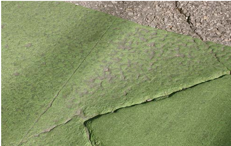
Figure B7. Thermoplastic thinning on the colored lane on San Jacinto Boulevard
