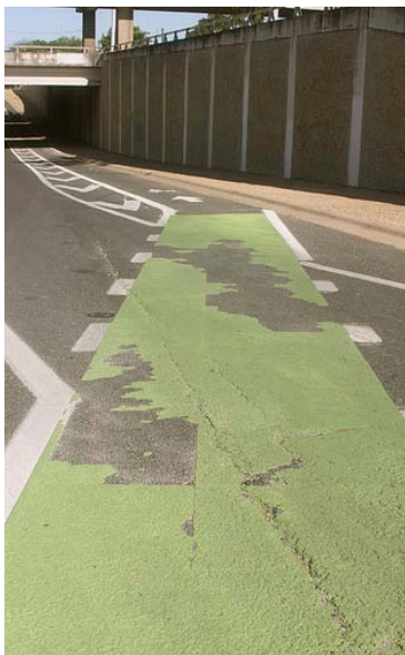
Figure B1. Deteriorating thermoplastic on one of the I-35 exit ramps (breaking up in sheets)
