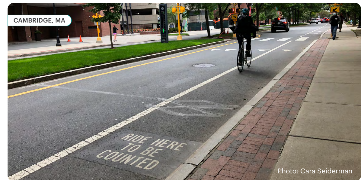
In-ground Inductive Loops installed in a bike lane.
