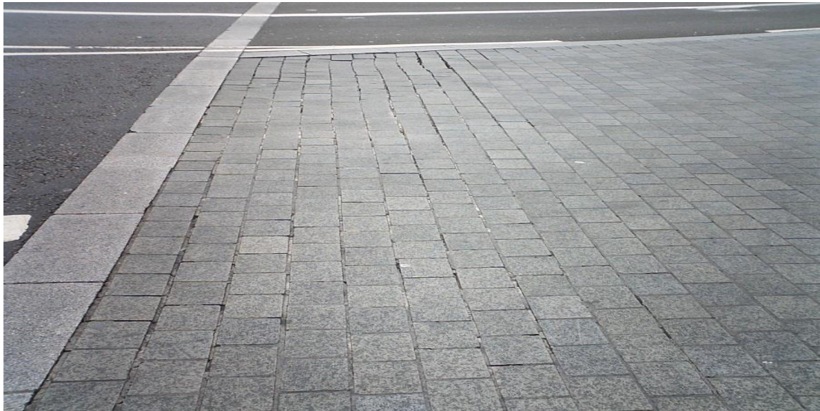
Picture 3 Stone Setts laid as rigid paving damaged kerb edge restraint
