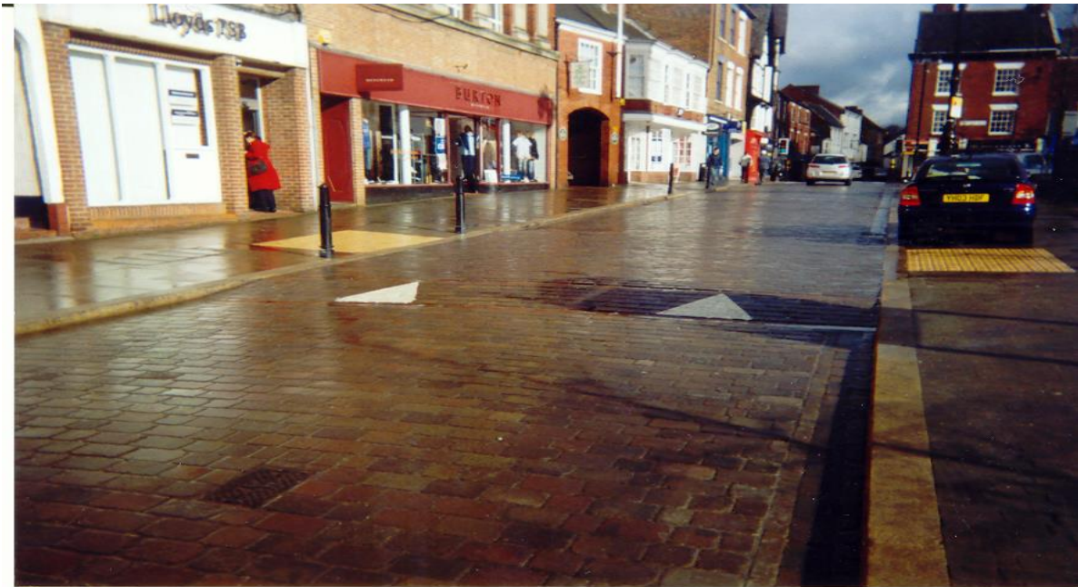
Picture 2 Tegula blocks laid as rigid paving damaged kerb edge restraint
