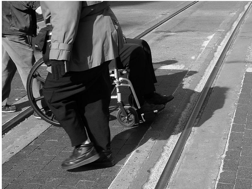
Figure 17 - Flangeway with excessive width that is incompatible with small wheels in a pedestrian crossing area.
