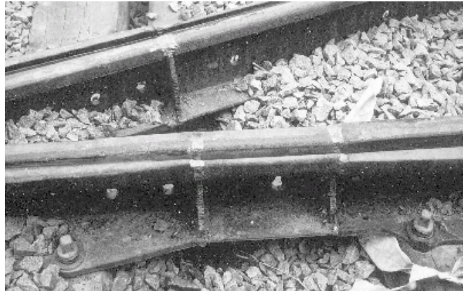
Figure 12. - Electrically welded connections between grooved rail sections and frog castings.
