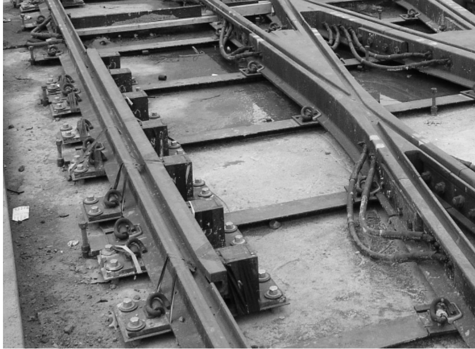
Figure 4. - The complex and expensive guard rail construction on tangent rail opposite the frog appears to provide no more useful guarding than the grooved rail itself would provide. Noteworthy is that in this instance the axles taking the diverging path through the frog are in fact guided by the grooved rail opposite the frog.
