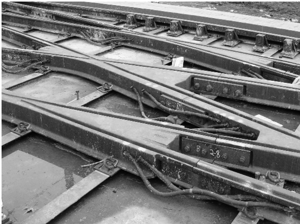
Figure 10. - Crossover consisting of grooved rail sections and castings, all bolted together.
