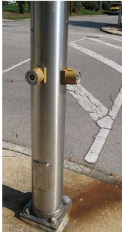
Push buttons without signs, even if functional, do not command the proper attention and respect from pedestrians.
