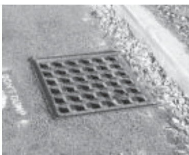
Parallel bar drain grates should be replaced with modern bicycle-safe and hydraulically efficient models such as the "vane" or "honeycomb" grates.
