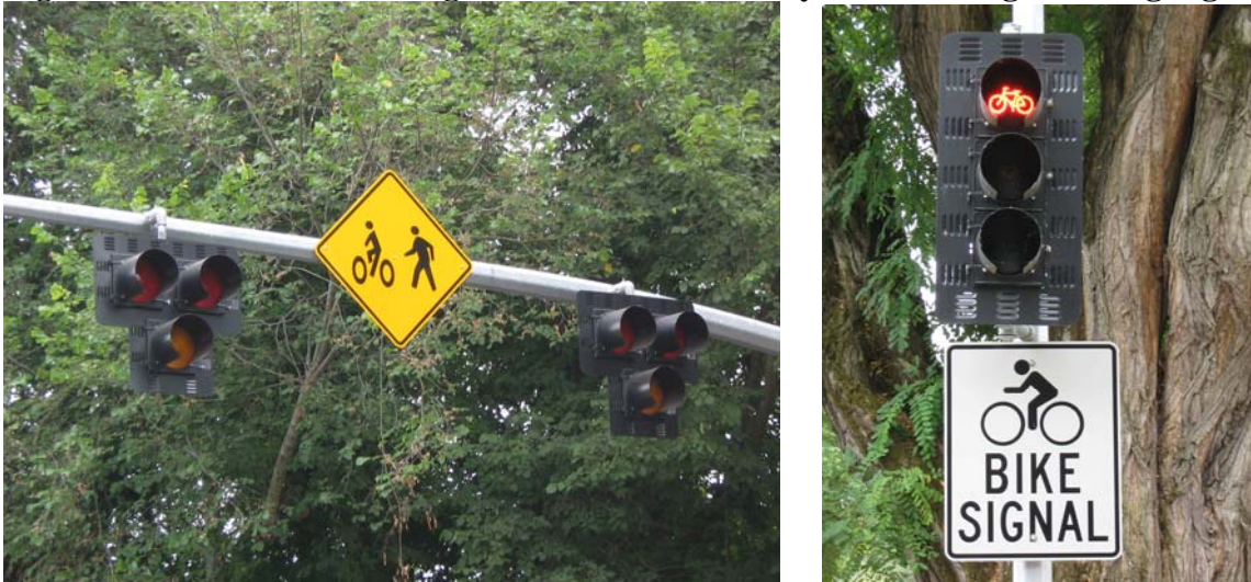
Figure 2: E. Burnside Bike Signal and Pedestrian/Bicyclist Crossing Warning Sign
