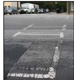
Faded pavement markings along Ponce de Leon Avenue.
