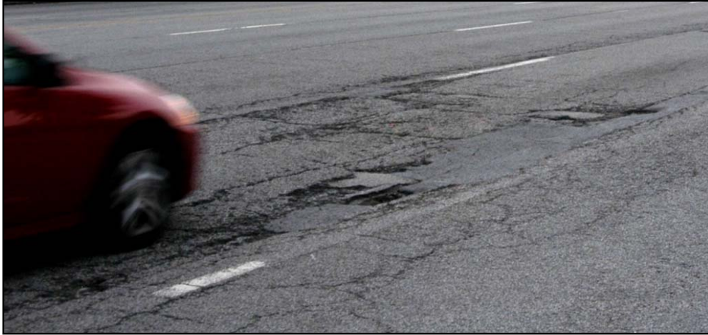
Potholes and cracks in the pavement along Ponce de Leon Avenue are potential safety hazards.
