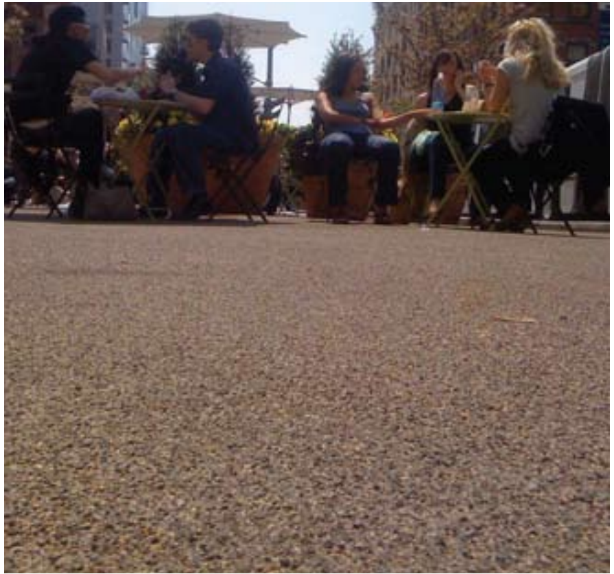
Resin-bound gravel treatment applied to existing asphalt roadway to create a temporary pedestrian plaza: 9th Avenue at West 14th Street, Manhattan
